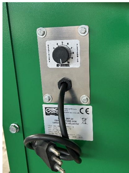
Fig. 2.3 – DEF variable speed drive
